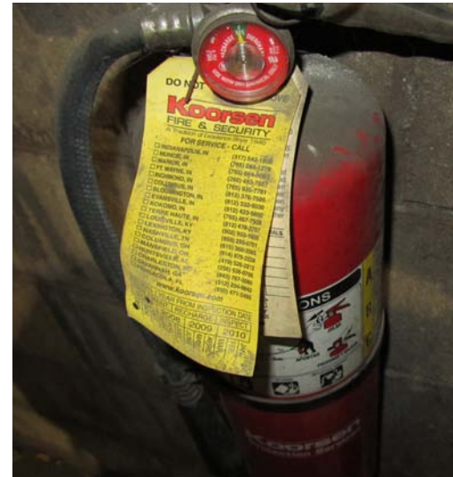
IOSHA Top Ten Most Violated Standards, number 9, Fire Protection: Fire extinguisher is nearly two years past the due date for the required annual service. (Photo taken by IOSHA Compliance Safety and Health Officer Jeanne Hedge)
