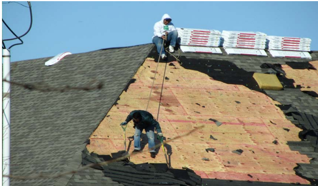
IOSHA Top Ten Most Violated Standards, number 6, Fall Protection: Employee is not properly protected from a potential fall. (Photo submitted to IOSHA)
